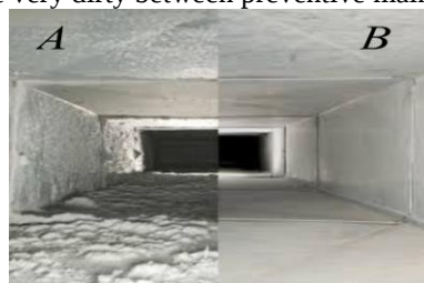
Figure 4. Air conditioning duct status A) dirty; B) clean
